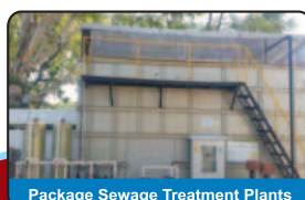
Package Sewage Treatment Plants
